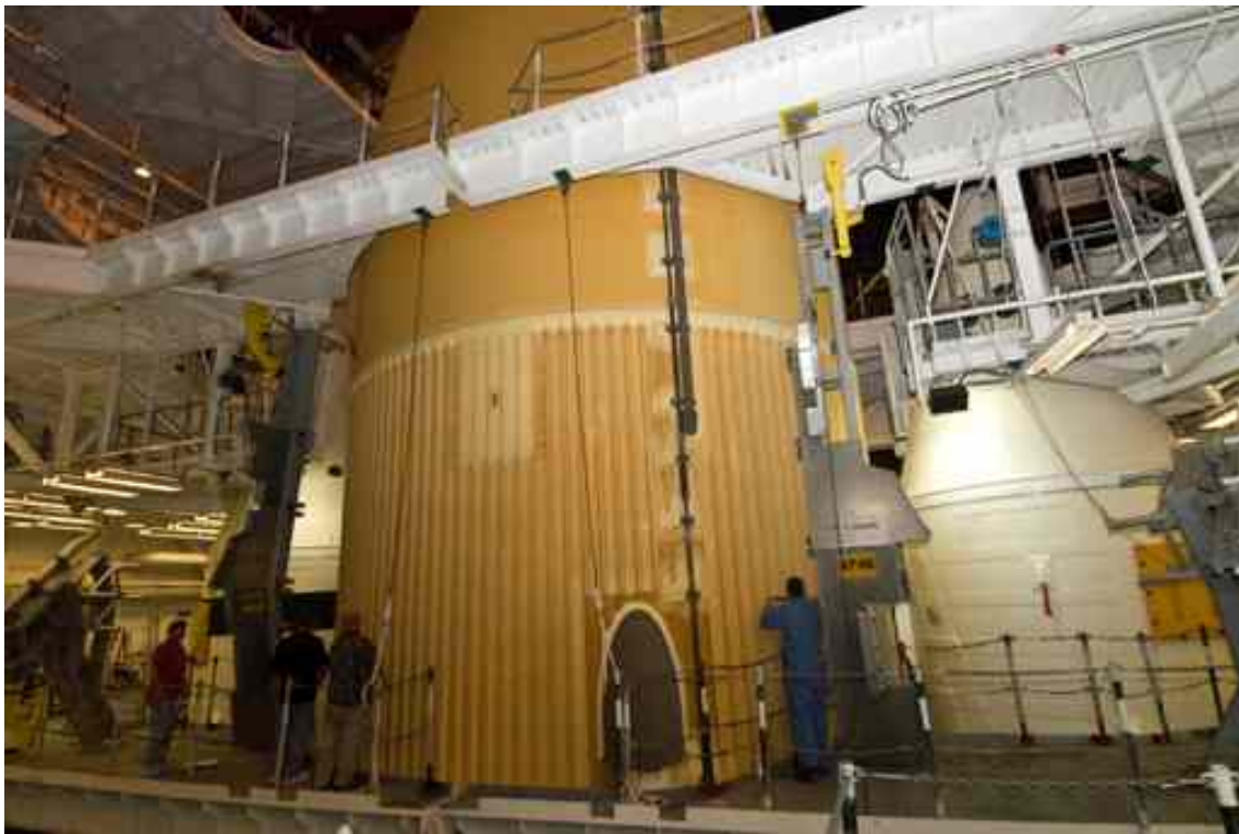
Engineers in the Vehicle Assembly Building test foam insulation on ET-132's central intertank.
